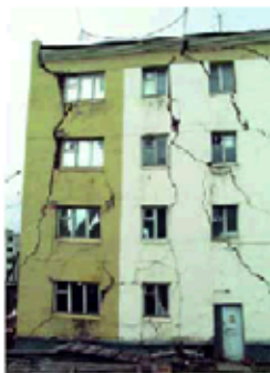
Building damaged due to permafrost thawing in Cherdyn (low Kibera River), Russia.
