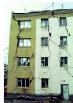
Building damaged due to permafrost thawing in Cherdyn (near Khatanga River), Russia.
