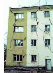
Building damaged due to permafrost thawing in Chersky (low Kolima River), Russia.
