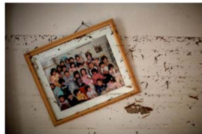
A picture frame and water marks are seen over the wall of a kindergarten destroyed by the earthquake and tsunami in Fukushima, northeast Japan, April 11, 2011. CREDIT: REUTERS/CARLOS BARRA
